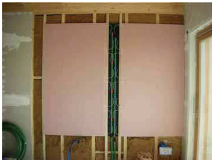
Fig. 11. Hydrothermal control system. The PCM Micronal panels contain microscopic capsules of wax that change phase between 22 and 26 ° C, accumulating latent heat and contributing to maintain internal temperature limiting overheating
