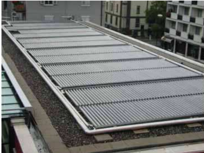
Fig. 10. Solar collectors system on the roof. It needs for hot water and heating. In the summer contributes to air conditioning inside the building.
