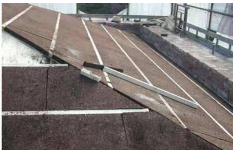
Fig. 7. Isolated and ventilated roof in historical building. The lack of adequate insulation causes excessive heat dispersion, the ventilation system favours a better summer behaviour.
