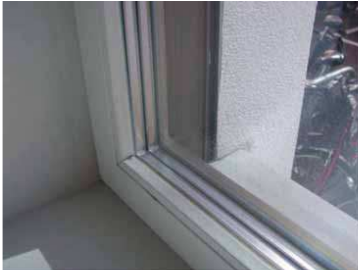
Fig. 12. External insulation. Detail of a window with triple glasses and double air interspaces
