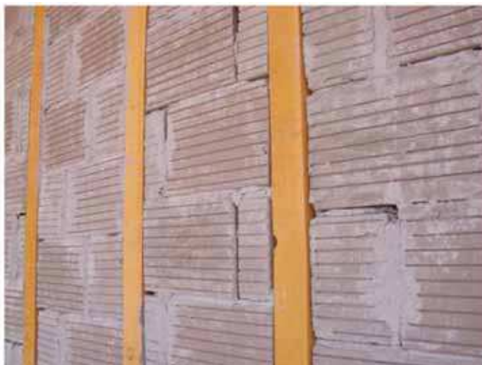
Fig. 6. The raw clay brick wall, with high heat capacity, helps to maintain equilibrium of humidity inside the building.
