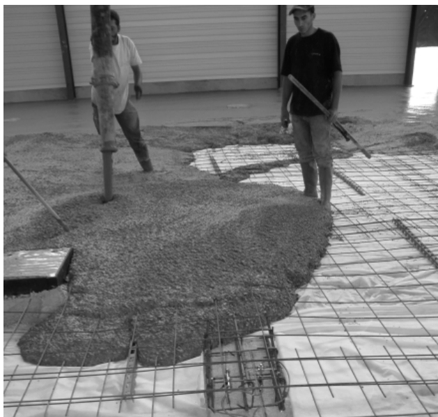
Fig. 10. Sensor cable must be robust: example of concrete pouring . Extracted from (Dubois et al., 2007)
