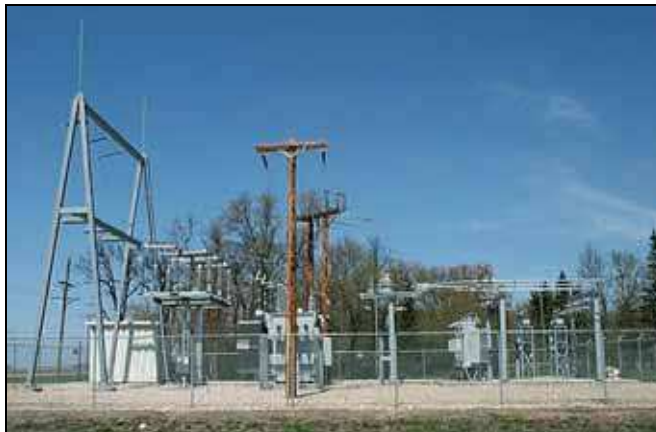
Fig. 1. Real electrical substation
