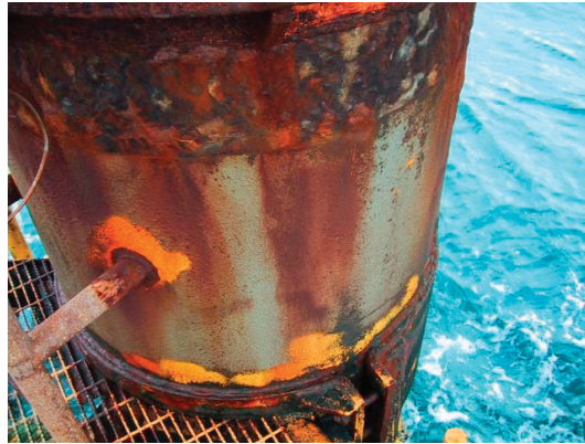
Figure 3. Degradation of offshore structural component [3].
