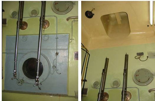
Fig. 3. Images from the Operator Room No. 4 (OR 4) serving the HC 4 [4]
