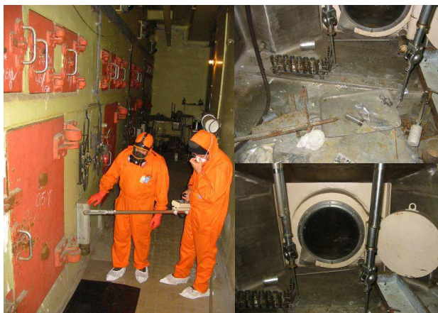
Fig. 4. Interior of the hot cell no. 4 (HC 4), opened in July 2006 [4]
