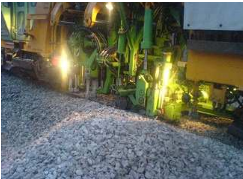
Fig. 17. Tamping and stabilizing operations after the installation of the railway track with B70-F sleepers (before the second stage of test)
