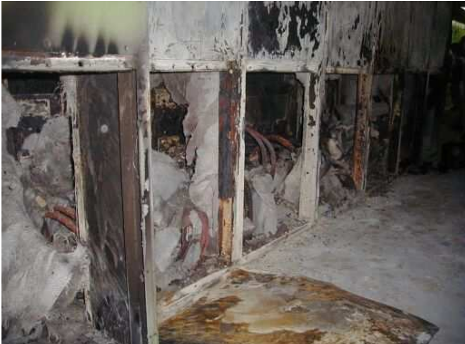
Fig. 4.3.2. Damage to the switchgear where the TP was connected.
