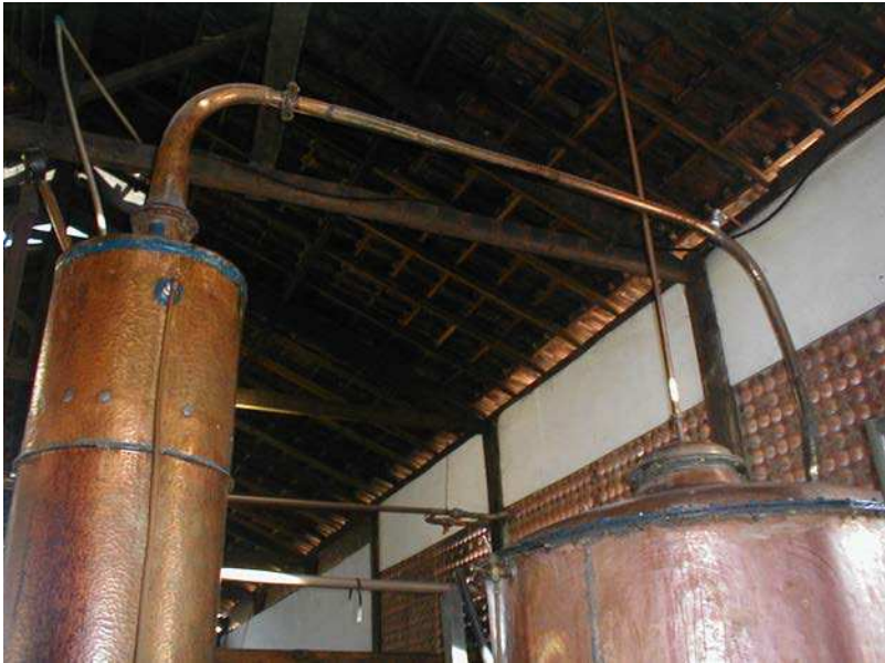
Fig. 11. Column (at the left) with temperature control by a tubular dephlegmator (alembic JLG ; Bemposta-RJ).
