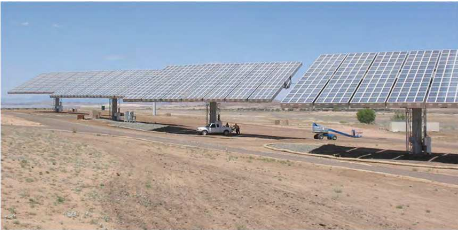
Fig. 2. Several 35-kW CPV systems built by Amonix in Torrance, California were installed at a Public Service power plant in Arizona. The system uses Fresnel lenses to concentrate sunlight onto high efficiency silicon solar cells. The pickup truck in the shade gives an idea of size of this installation.
