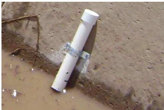
Fig. 7. Installed Hobo Pressure Transducer
