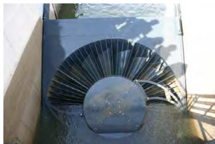
Photo 20. L'Ame: upstream view of the turbine.
