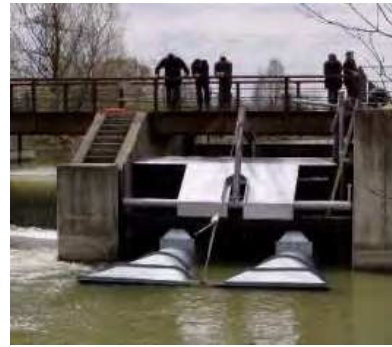
Photo 4. Marchfeldkanal: the turbines.
