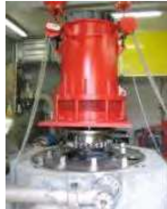
Photo 8. Le Châble Profray: The turbine and its runner and the alternator, during the erection.
