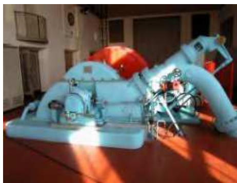
Photo 2. Mühlau: Drinking water turbine (2-nozzle Pelton turbine).
