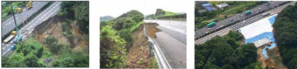
(a) Overview of sliding (b) Shoulder and slope slid (c) Urgent retrieval
