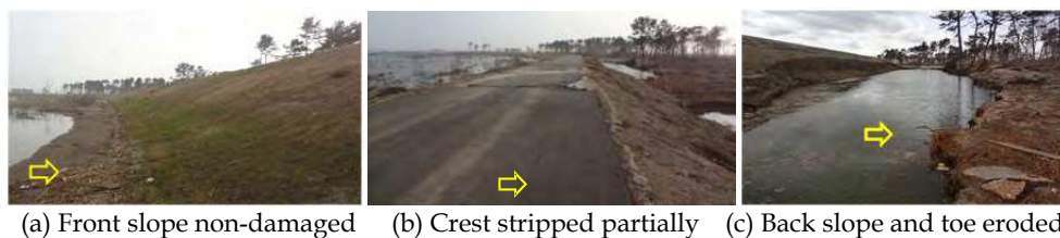
Photo 8. Dyke overflowed by tsunami
