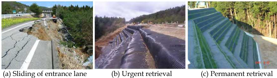
Photo 4. Damage and seismic retrieval with geotextile
