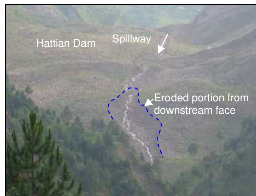
Fig. 7. Front view of the Hattian landslide mass, showing the downstream face erosion.
