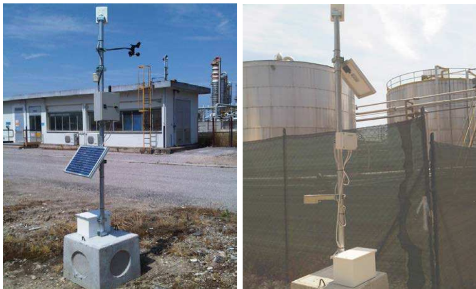
Fig. 6. SN (left) and EN (right) units installed in proximity of the pipeline and of the chemical plant
