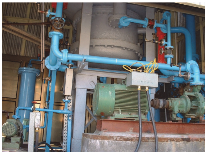
Fig. 3. Evaporator section of Desalination unit and Booster pump
