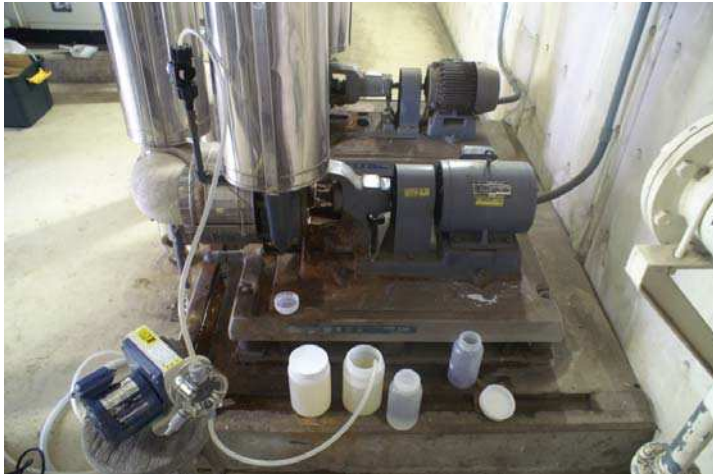
Fig. 16. Addition of LSP-01 from the discharged side of the main pump
