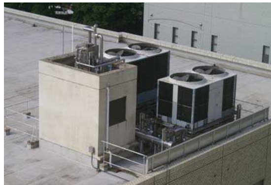
Fig. 14. Heat pump - chiller units
