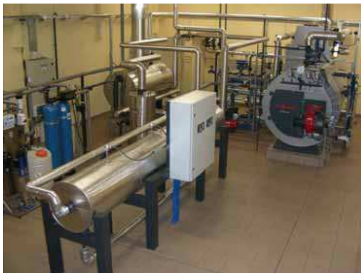
Fig. 11. View of the experimental installation for testing the computer system for on-line monitoring thick-wall pressure components
