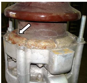
Fig. 2. Corrosion in the metallic parts of the surge arrester.
