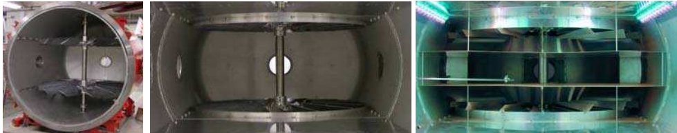
Fig. 6. Photographs into the flow generation section of the AWTS-II facility, Left shows the 1.8m diameter fans installed, Center shows with the upper and lower flow separators and Right the system of vertical and horizontal flow guides compartmentalizing the flow, preventing rotation and excessive turbulence.
