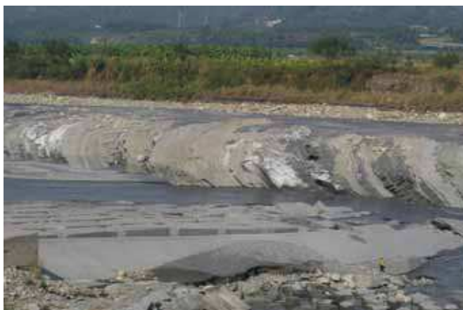
Fig. 14. Scoured channel bed downstream of the Chi-Chi Weir
