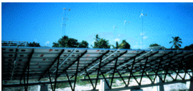
Fig. 14. Xcalak, Mexico wind turbines and PV array (1993).
