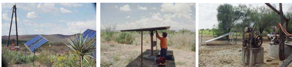
Fig. 4. PV water pumping systems in Chihuahua and Baja California Sur, and FIRCO engineer conducting performance evaluation.
