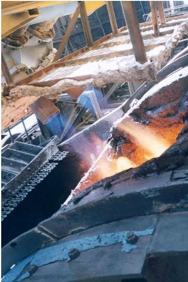
Fig. 7.1 Photo of Burners Installed in P&S Furnace
