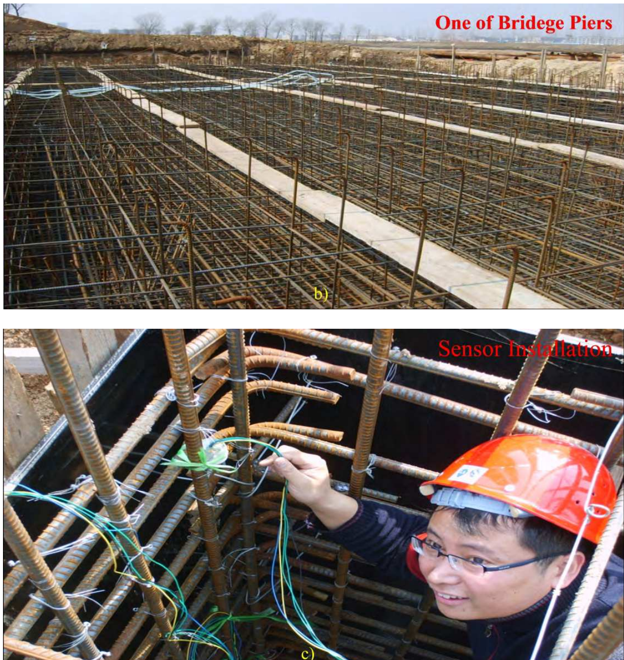
Fig. 32. Corrosion monitoring of the bridge pier. Scheme of the sensors' location a), Bird's eye view of the pier b) , and the sensor installation c)
