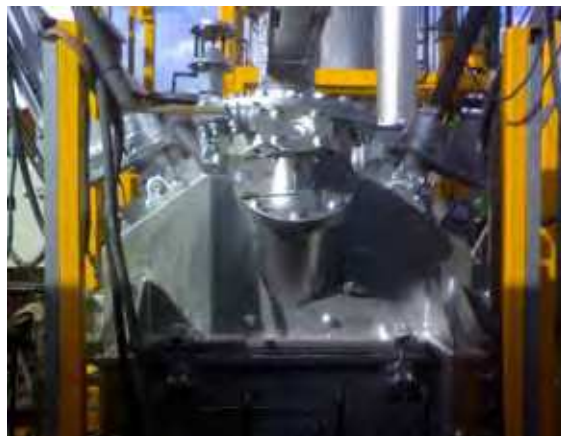
Photo 7. Gasification / vitrification furnace
