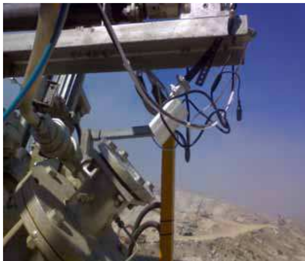
Photo 10. Camera recording what is happening in the furnace
