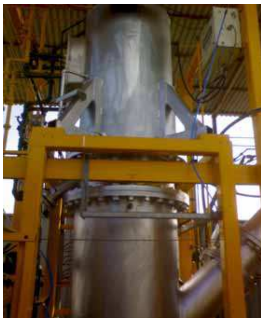
Photo 17. Secondary Combustion Chamber
