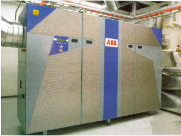
Figure 4. Prototype Ingersoll-Rand Power Works™ installed on Jamacha Landfill - United States.
