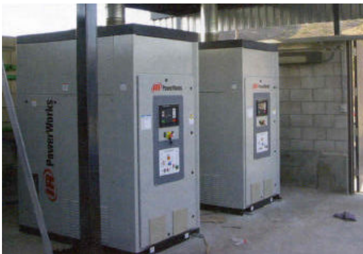
Figure 3. Ingersoll-Rand Power Works™ installed on the Jamacha Landfill - United States.
