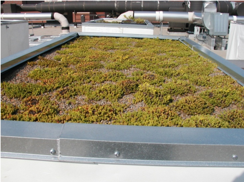
Figure 9. Vegetative mini-roof equipped with sedum plants.
