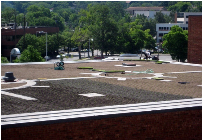
Figure 13. Construction phase for installing a pilot vegetative roof on top of Hulsey Center.
