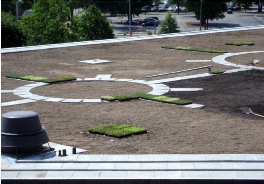
Figure 12. Construction phase for installing a pilot vegetative roof on top of Hulsey Center.
