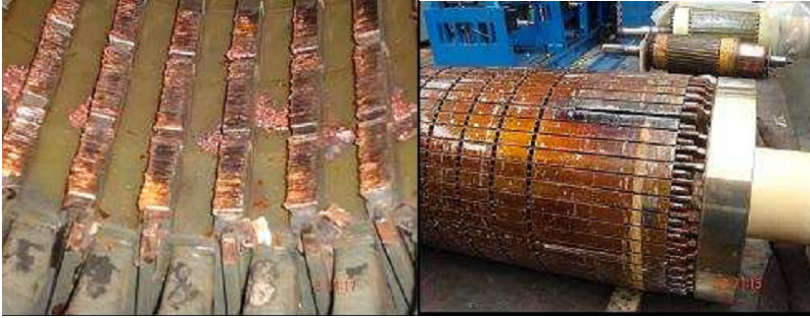
Figure 26. Stator and Rotor Damages
