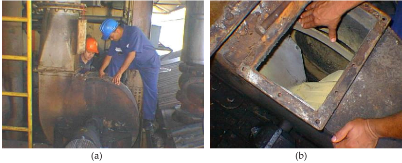
Figure 7. Photos of the attack-sites of samples: a) Ventilator extractor where samples were placed, b) Ventilator damp where samples were anchored.
