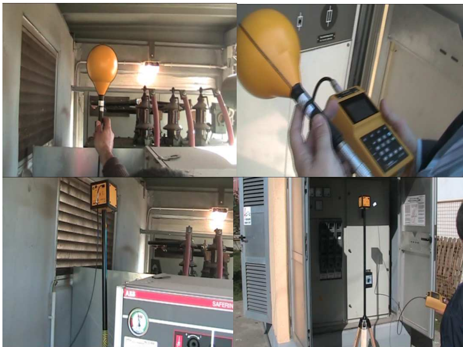
Fig. 15. The measurement of magnetic and electric fields in KBTS 10(20)/0.4 kV
