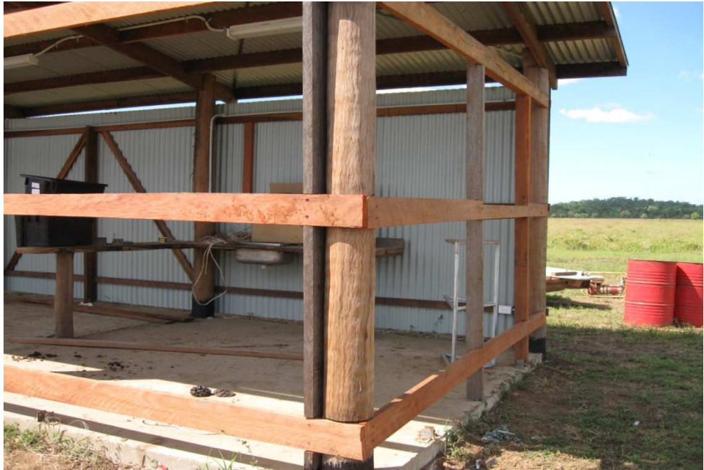
Fig. 4. The Kitchen Unit Showing Construction of Traditional Log Columns and Milled Timber Girts
