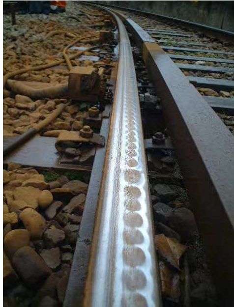
Fig. 2. Example of rail corrugation
