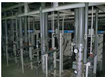
Fig. 9. Pleiade® MBR membrane bioreactor for treating 1000 m 3 /day of effluent from www.vic-ws.it/site/down/PLEENG0411.pdf
