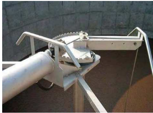
(b) Cable and gear protection system
