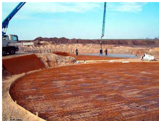
Fig. 8. Structuring the grid irons for a commercial biogas plant (MT-ENERGIE GmbH & Co. KG)
