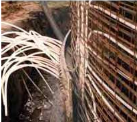
Fig. 13. Integrating the heating tubes (BIOGAS NORD GmbH)
