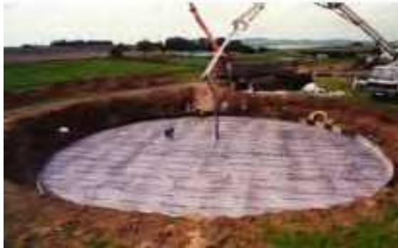
Fig. 9. Pouring the concrete mixture for a commercial biogas plant (BIOGAS NORD GmbH)
