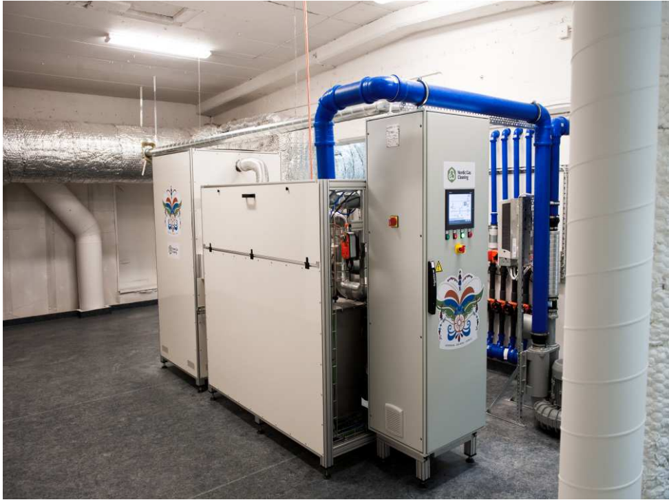
Fig. 4. The unit from NGC installed at Södertälje hospital. (Photo Anette Andersson)
