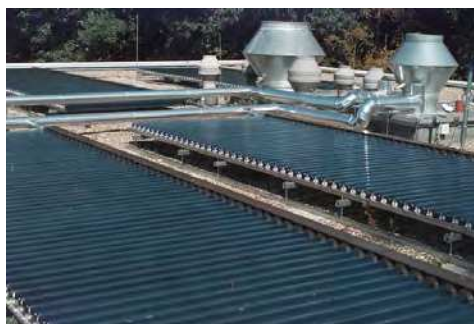
Fig. 19. Solar collector field (evacuated tubes) installed in system at University hospital in Freiburg (Henning, 2007).
