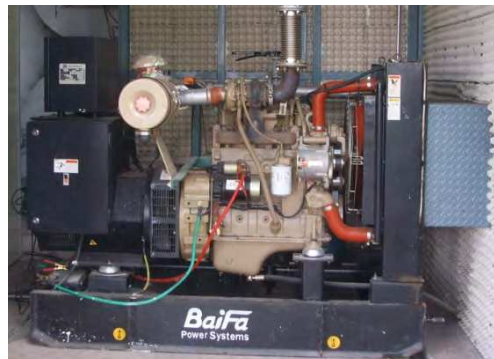
Fig. 16. Internal combustion engine-generator for power generation
