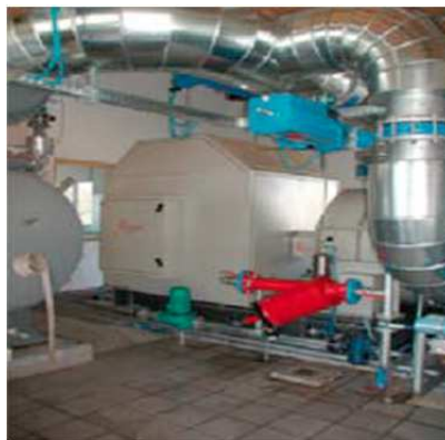
Fig. 1. Photograph of Altheim geothermal binary power plant in Austria (Ruggero Bertani, 2007).
