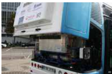
Fig. 2. Detail on fuel cells, the ESS is composed of Li-ion battery and supercapacitors (TriHyBus.cz, 2008)
