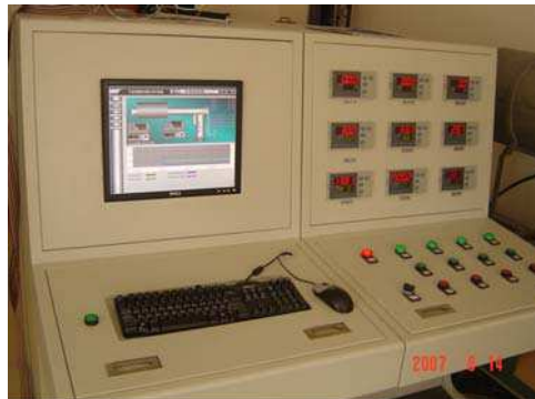
Fig. 12. Monitor equipment of heat pipe technology
