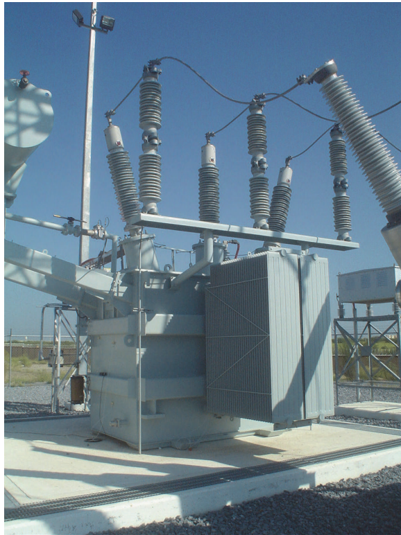
Fig. 3. Power transformer at the electrical substation. (Courtesy of Prolec GE ).
