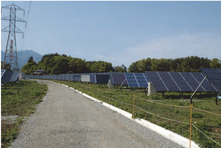
Fig. 4. The 2 MW Hokuto mega-solar plant
