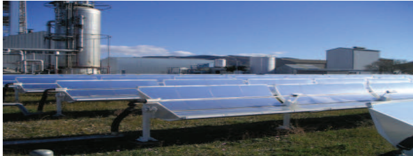
Fig. 23. ACUREX solar plant
