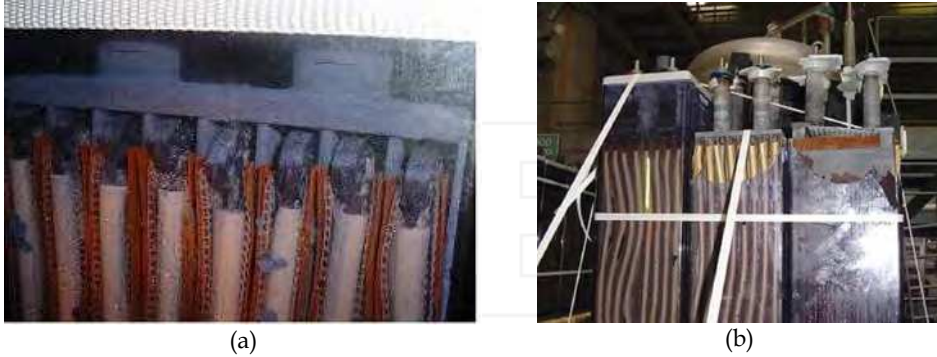
Fig. 5. Due to corrosion, short-circuit took place and caused explosion accident in a standby tubular battery: (a) positive plate lengths were increased and touched the negative collective bar, (b) positive plates were distorted; the positive terminal obviously became more higher than the negative terminal; battery was destroyed after explosion (Source: EDF)
