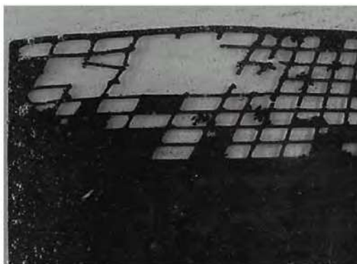
Fig. 6. Corroded positive plate of a starter battery, at the end of 5 years of service life in a passenger car (Ruetschi, 2004)
