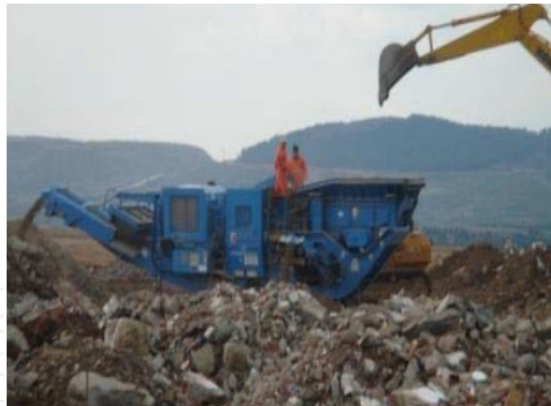
Figure 3. Demolition Waste Recycle Facility [35]
