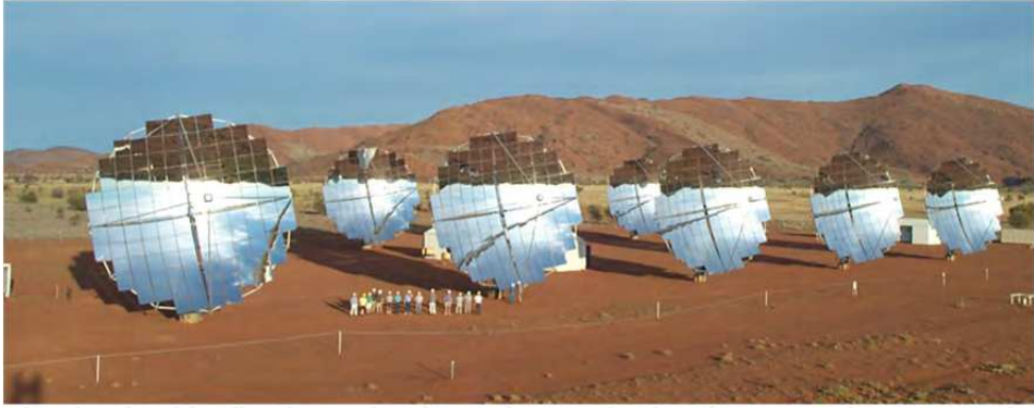
Fig. 3. Several 25-kW CPV systems built by Solar Systems in Hawthorn, Australia, and installed on aboriginal land. These systems use mirrors for concentrating sunlight onto silicon solar cells---see www.solarsystems.com.au The people in the foreground give an idea of the system's size (photo by R. McConnell).
