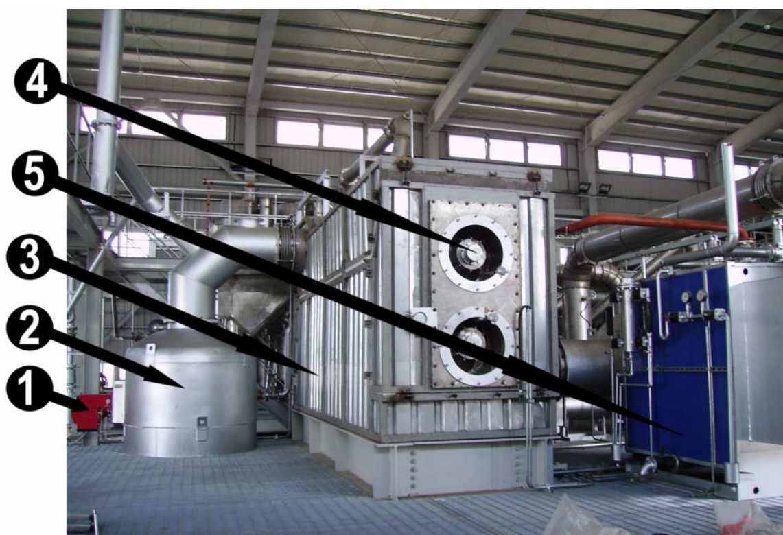
Pict. 1. ENRESTEC thermal units for waste tire pyrolysis with steam: 1 – oil fuel burner, 2 – furnace, 3 – pyrolysis reactor heating box, 4 – double-screw reactor in the box, 5 – second heat steam boiler.
