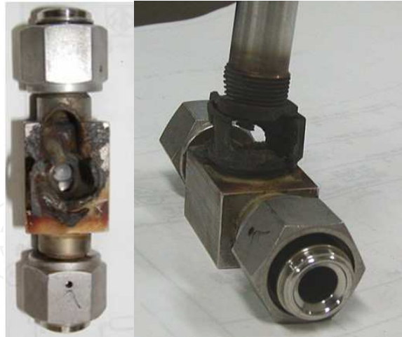
Fig. 5. A burnt valve in a nitrogen trifluoride line caused by adiabatic compression.
